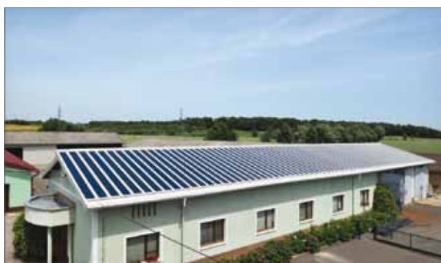
FIG. 15: RATED POWER OF THE PV POWER PLANT: 10 kWp
